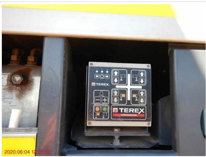
Outrigger Controls and Labeling
