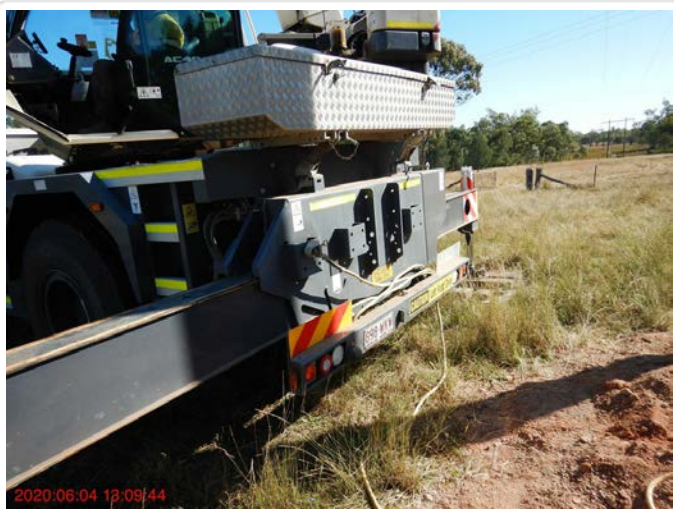
Appropriate Earthing Supplied and fitted by trained high voltage linesmen
