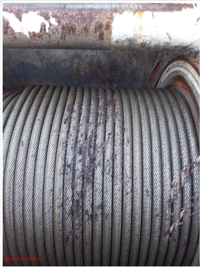
Main Wire Rope
