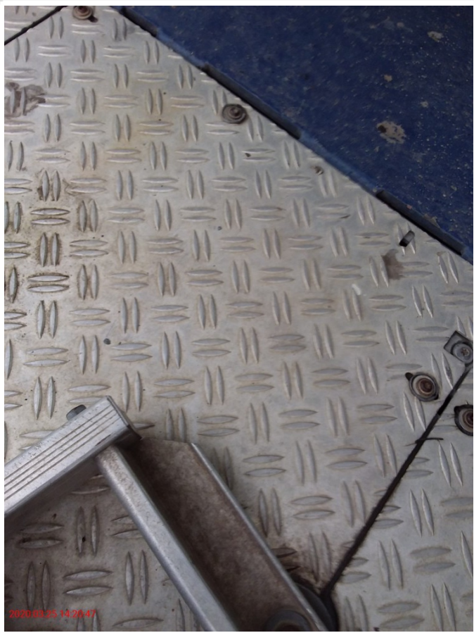
Return Filters and Housing Under the cover
