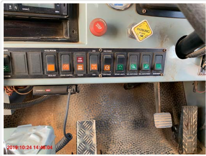
Switches and Relays
