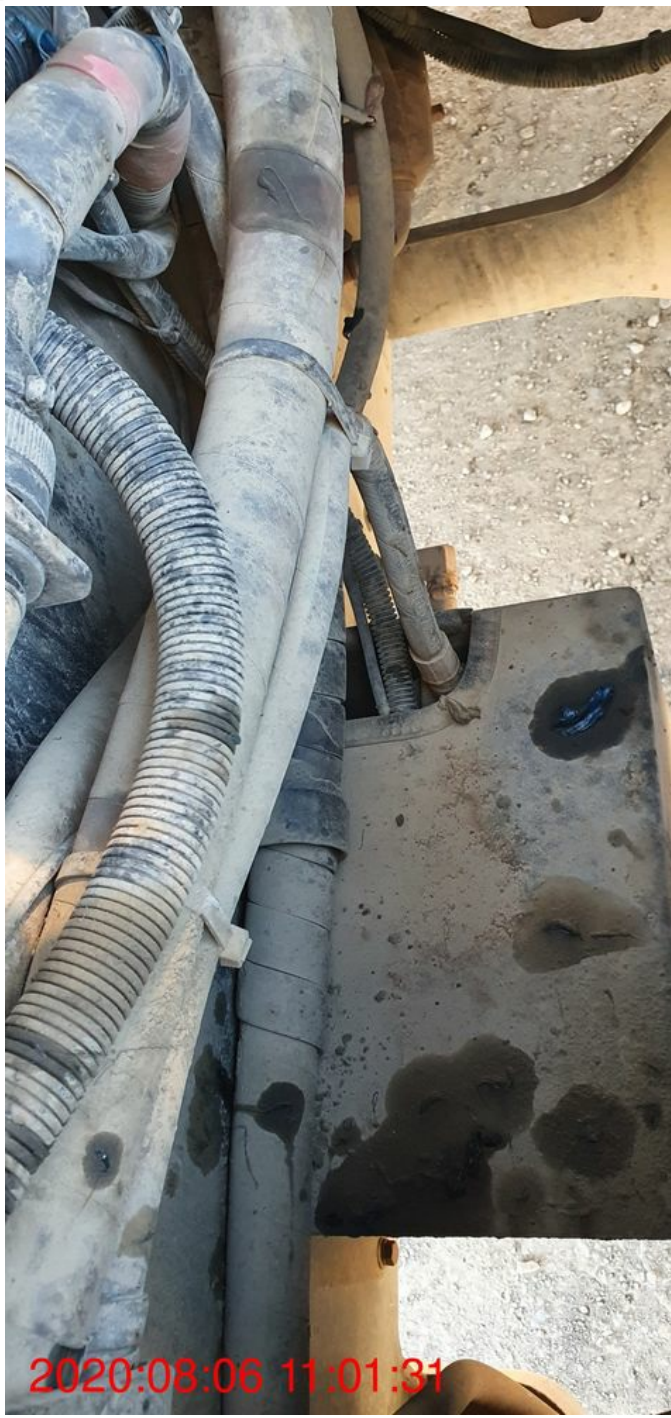
Emergency Steering Pump
