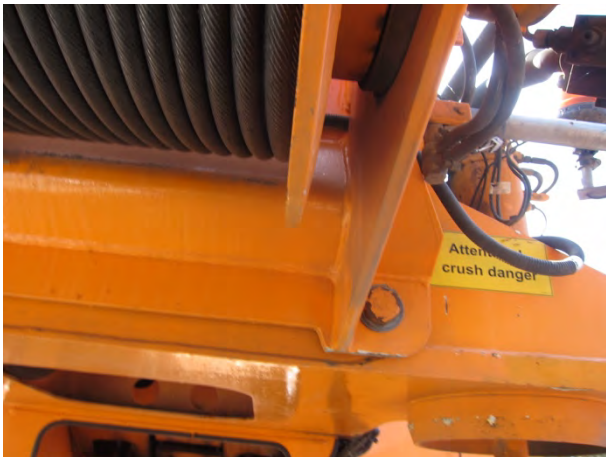
Photo 11: Winch sheave mount
