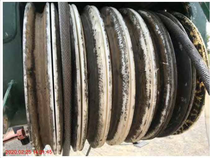
Head Sheaves and bearings
