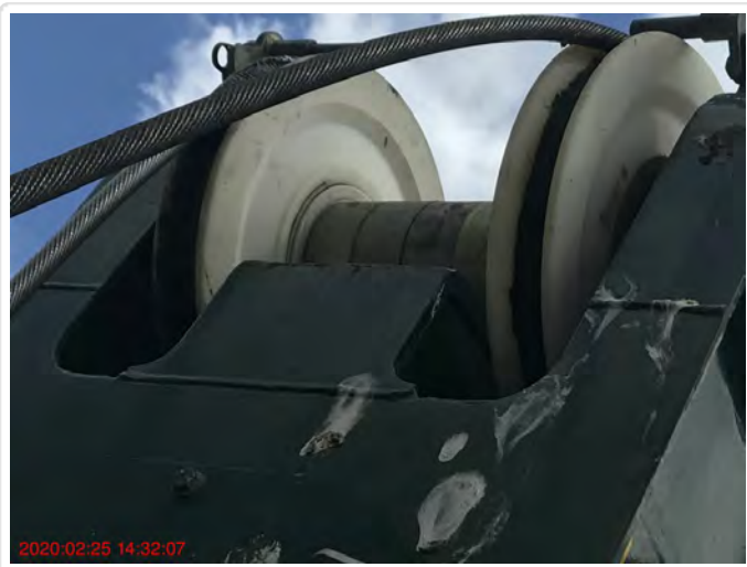
Idler Sheave and Bearing
