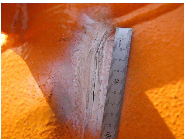
Photo 19: Crack on right side turret weld
