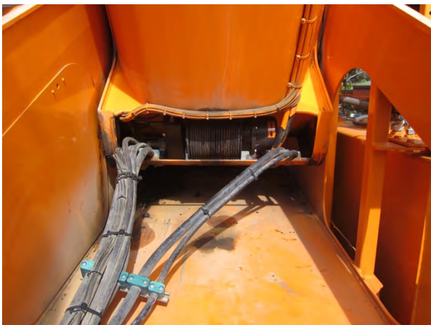
Photo 7: Internal turret and boom welds
