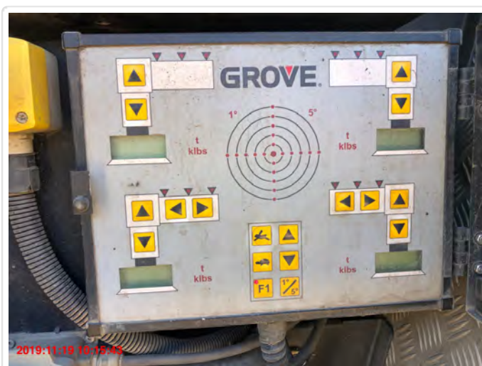
Outrigger Controls and Labeling
